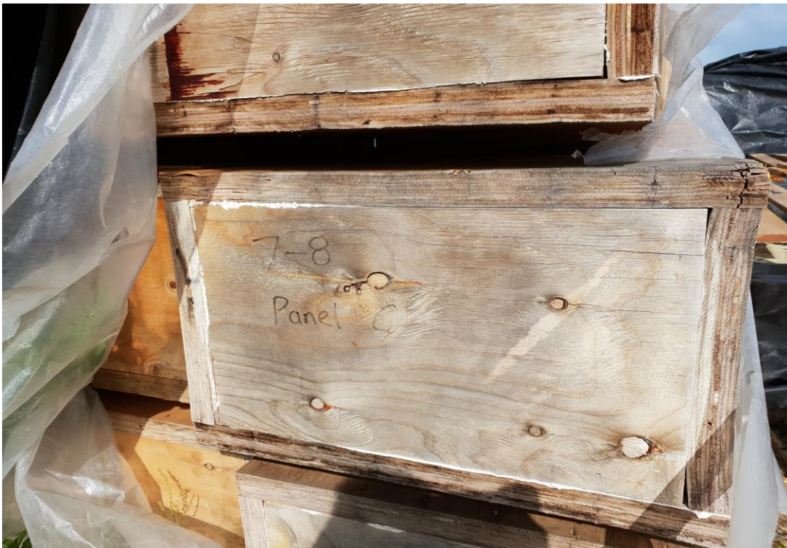
Figure 5: These Potius Panels have had long term exposure to weather resulting in swelling, discolouration and some splitting.
